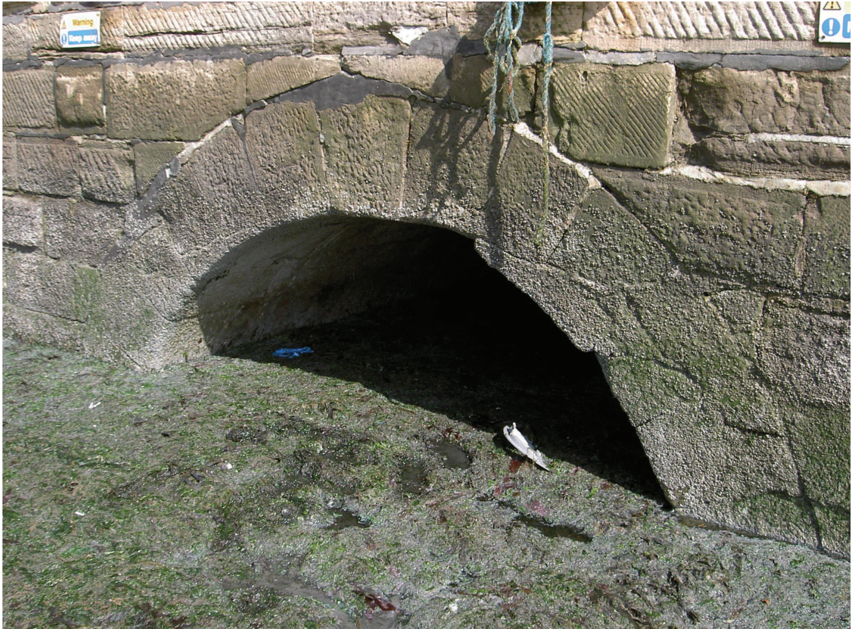
Margate Harbour Sluice –open end of culvert viewed from inner face of Stone Pier
